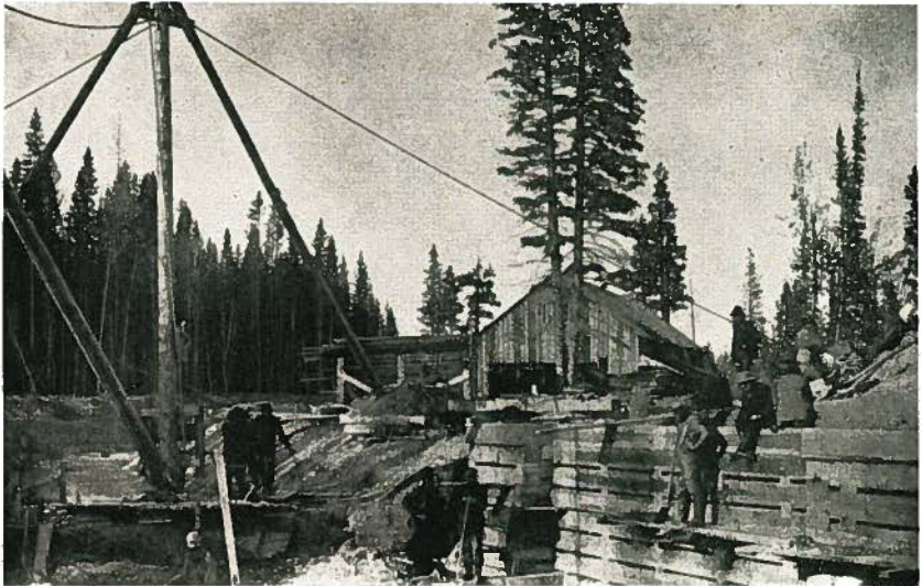
(Courtesy Vice-Admiral H. T. Baillie-Grohman, C.B., D.S.O., O.B.E.) Kootenay Canal at Grohman (Canal Flat), showing the lock under construction, 1888.
