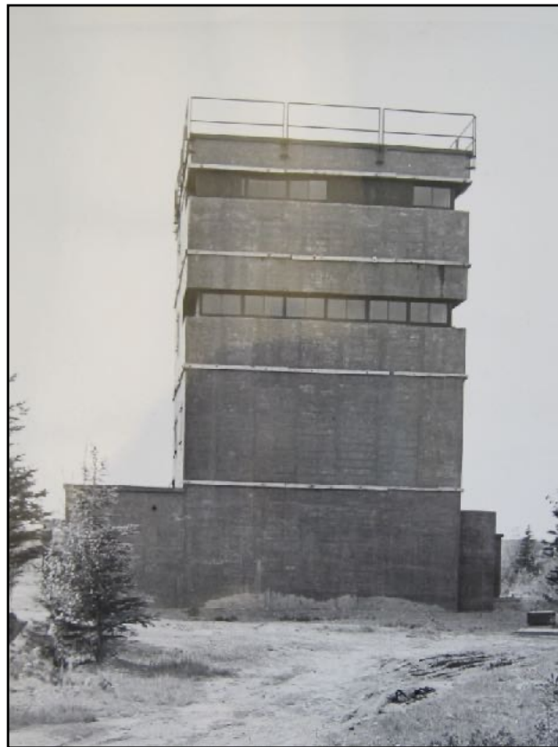
The Battery Observation Post under construction at Oxford Battery. Oxford Battery Fort Record Book.
