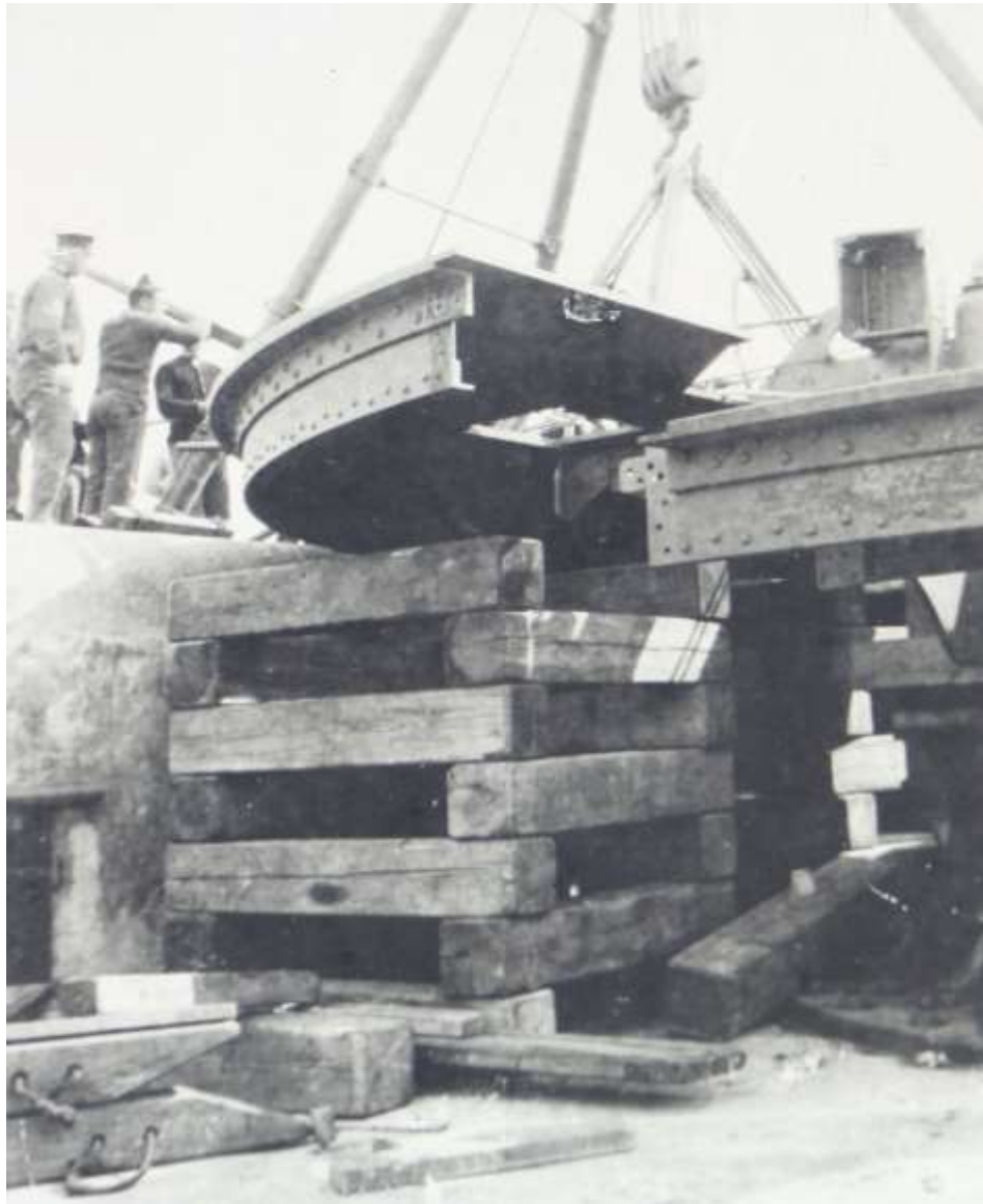
Erecting a 9.2-inch gun platform at Signal Hill Battery (Rodd Hill National Memorial archive)
