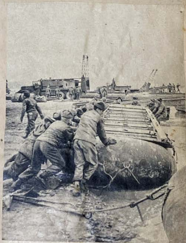
BLOWING UP and launching pontoons is one aspect of a bridging operation or of landing supplies on a sea beach. It is now the rainy season in North Korea and these kinds of jobs are complicated by heavy rains, swollen rivers and mud.
