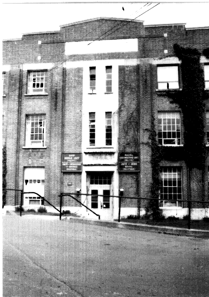
5 Building D192, main (southern) elevation, detail of brick and stonework. ( Ian Doull, AHB, Parks, 1989. )
