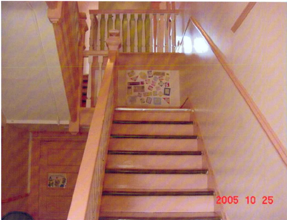
Figure 8. Main staircase, WP1163, Military Family Support Centre, Work Point Barracks, CFB Esquimalt (DND, 2011).
