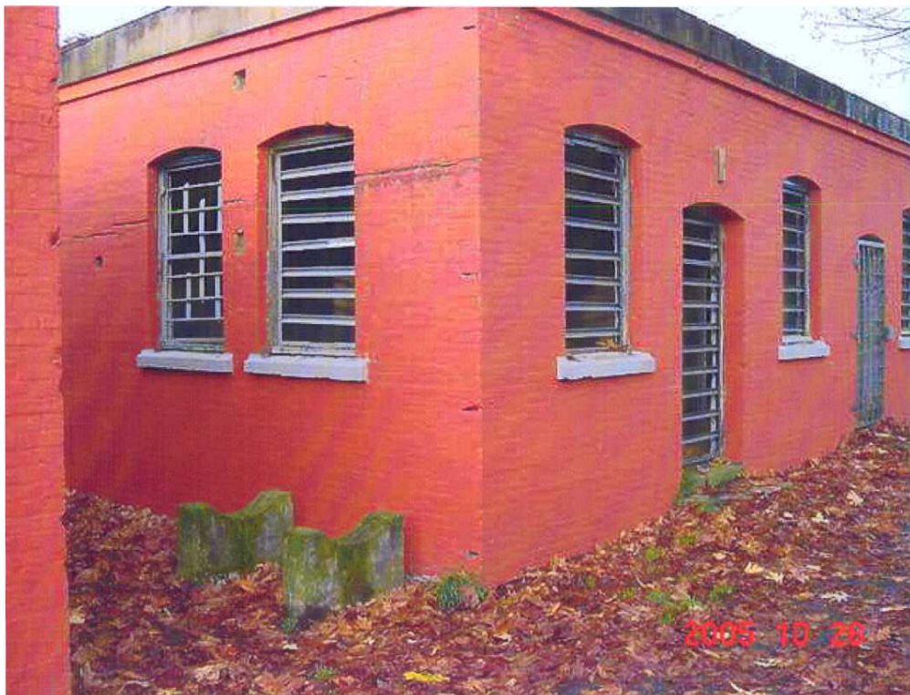
Figure 27. South and front elevations, WP1200, Artificer's and Fitter's Shops (Ian Doull, Parks Canada, 2011).
